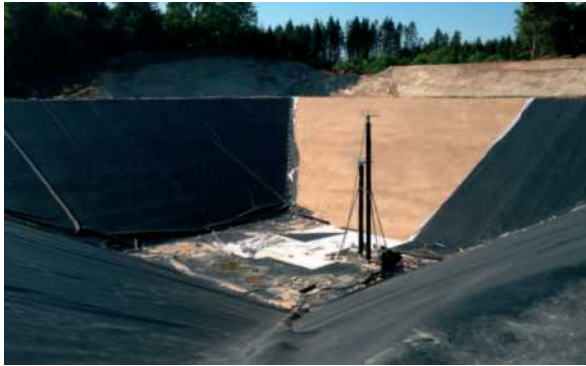
Figure 11: A 60.000 m 3 seasonal storage in the construction phase. located in Dronninglund, Denmark
