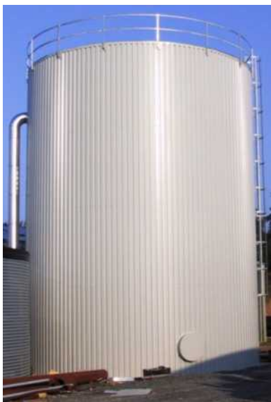
Figure 9: A cylindrical daily storage tank
