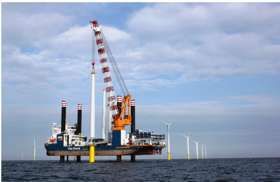
Figure 6: The installation vessel of the Saint-Brieuc project, the Aeolus ( Van Oord , 2020d)
