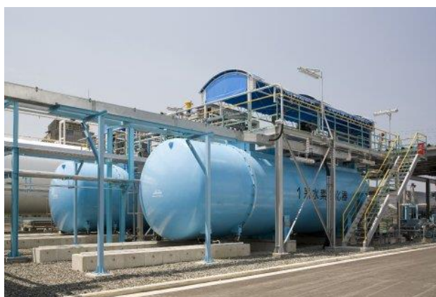
Figure 11 - Cryogenic liquid hydrogen tanks. Source: (US Department of Energy n.d.)
