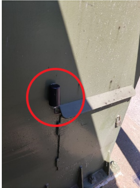
Figure 13: The antenna is installed outside the metallic enclosure.
