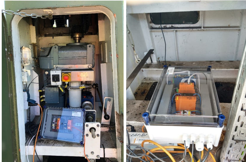
Figure 12: In the right image from top to bottom the industrial router, diagnostic equipment and the power supply is shown. On the left image, the power supply and diagnostic equipment are shown inside the DIN rail enclosure box (the industrial router was not yet installed).
